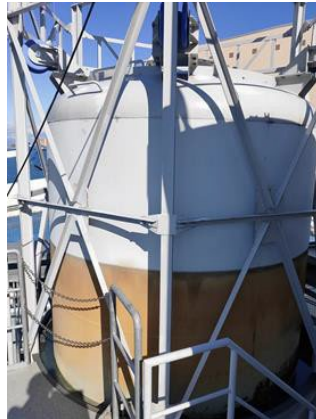
Biogas recovery tank
