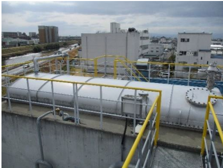
Wastewater treatment plant Anaerobic treatment tank
