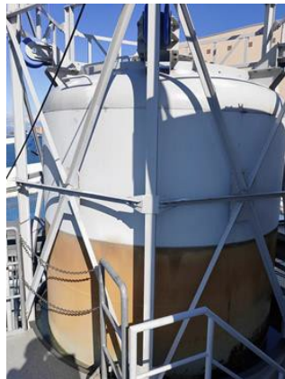
Biogas recovery tank
