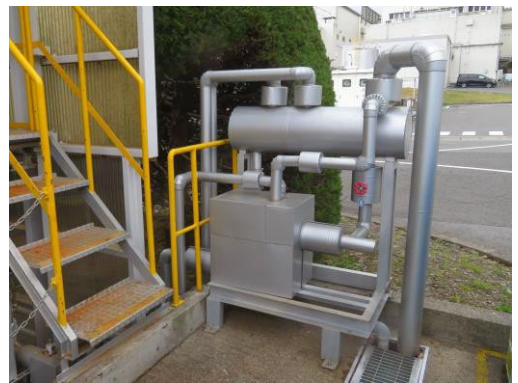
Waste heat recovery from sludge dryers
