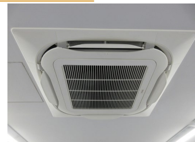
Air-conditioning systems using alternative CFCs
